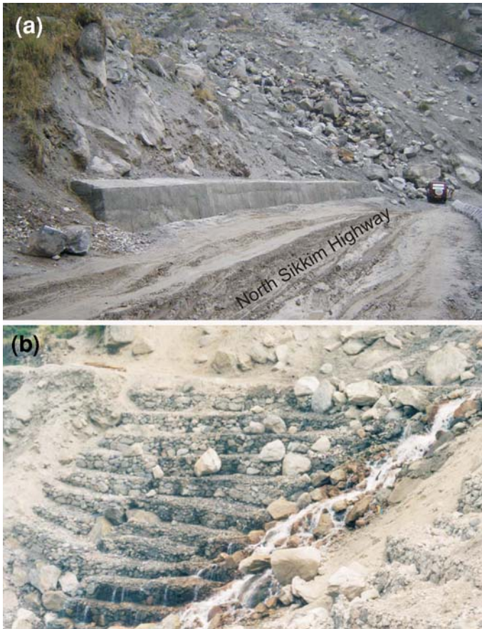
Fig. 2 a A view of the Lanta Khola Landslide at and above the Road (NSH) Level. Note the preponderance of boulders and debris material. b View of the Lanta Khola slide below the Road Bench. Note the remains of the gabion walls used for the slope protections during earlier remedial measures
