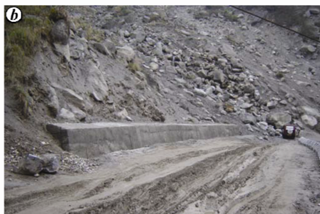
Figure 2. a , Location of the Lanta Khola Slide in Sikkim; b , A view of the Lanta Khola Slide from the road level.
