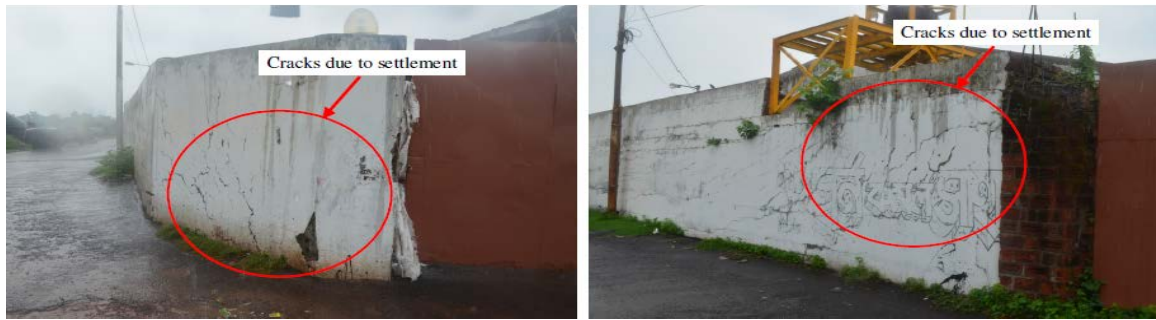
Figure 3. Structural distress due to differential settlement in facilities constructed over Dhapa Landfill
