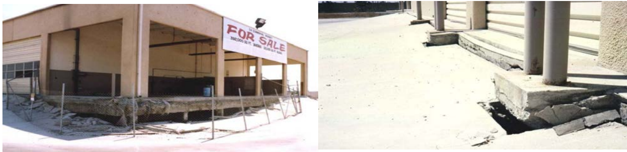
Figure 4: Differential settlement and distress in facilities constructed over inactive MSW landfills (source: http://www.scsengineers.com )
